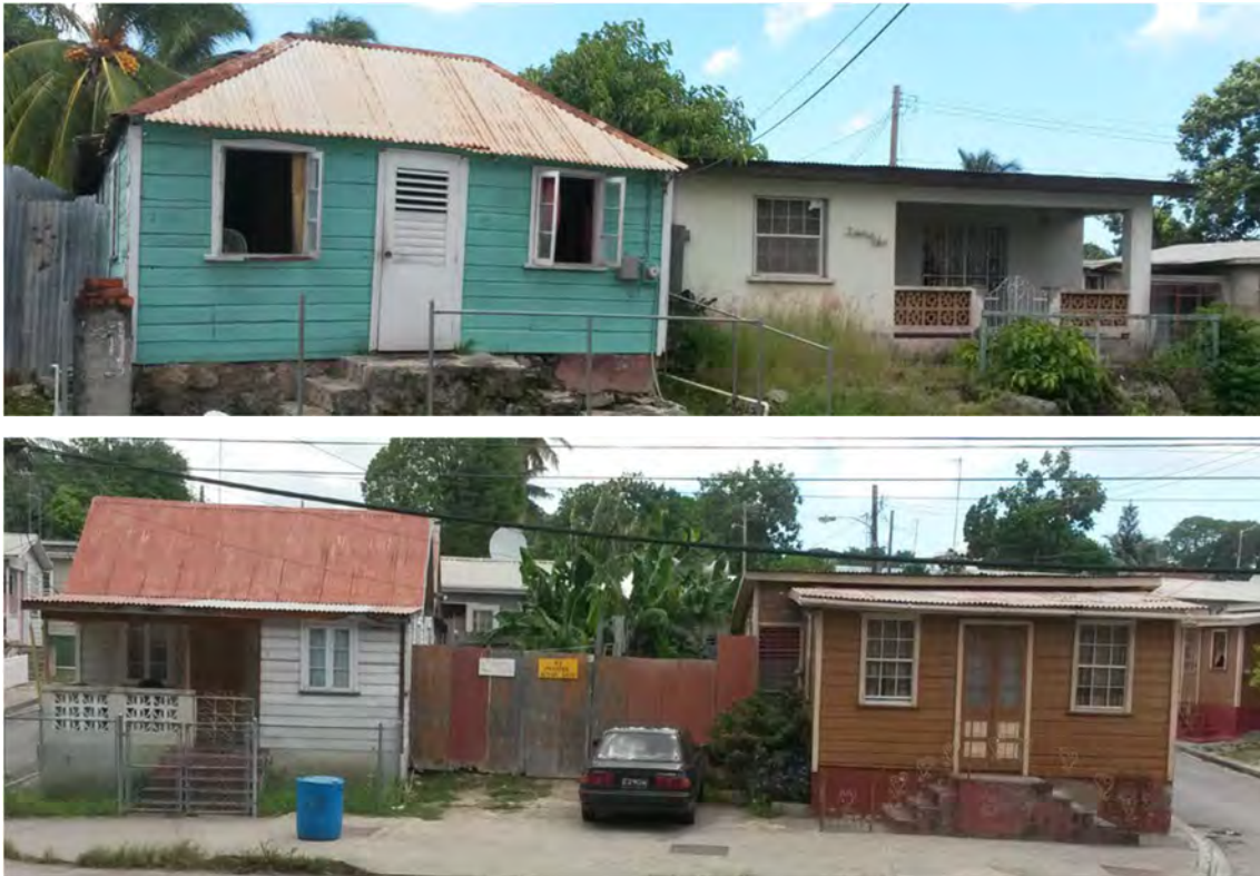
Figure A.35. Roof Types from Field Survey. Clockwise from top left: Hip, Flat, Lean-to, and Gable. (Source: Baird, 2017b).
